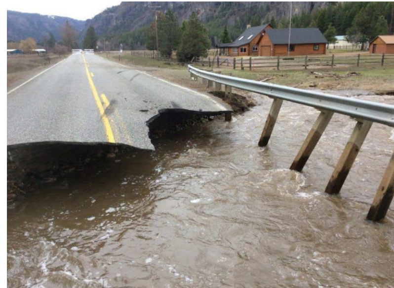
April 2017 flooding in Washington State, Credit: WSDOT
